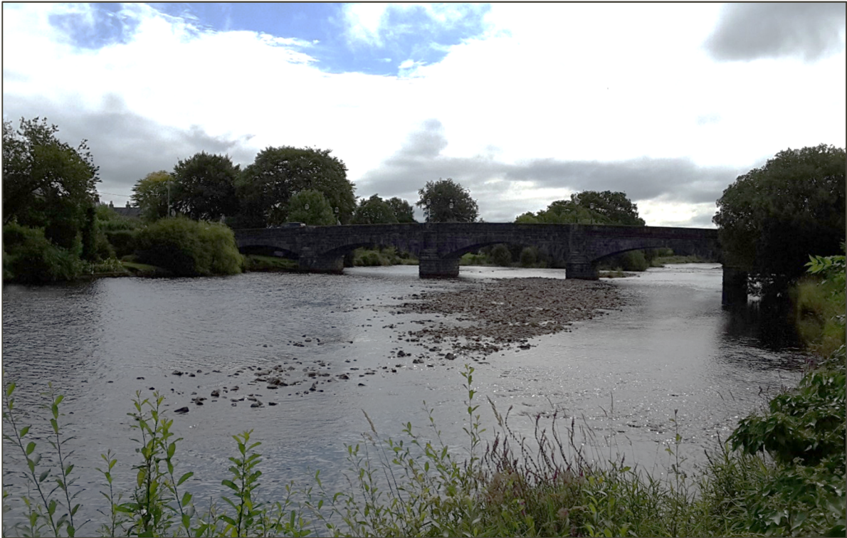
Figure 2. 6 Cree Bridge taken from upstream looking downstream. A large depositional bar has been deposited upstream of the bridge.
