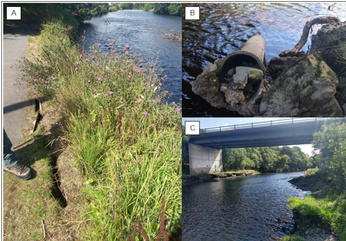
Figure 2. 8 River Cree, close to A75 road bridge (A) Tension crack along the footpath at the top of the right bank, upstream of the bridge. (B) Failed outflow pipe on the right bank under the A7 bridge. (C) Scour under the A75 road bridge (taken from the upstream of the bridge, looking downstream).
