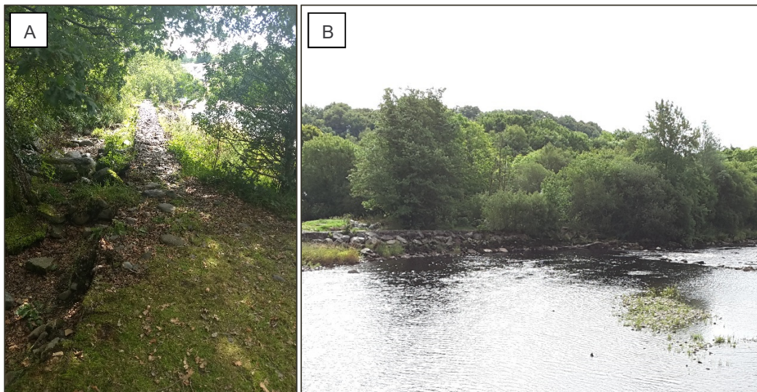
Figure 2. 5 (A) Rock mattress reinforcement on the surface of the made-ground behind Mill island. (B) Rip-rap revetment on the left bank of the made-ground behind Mill island.
