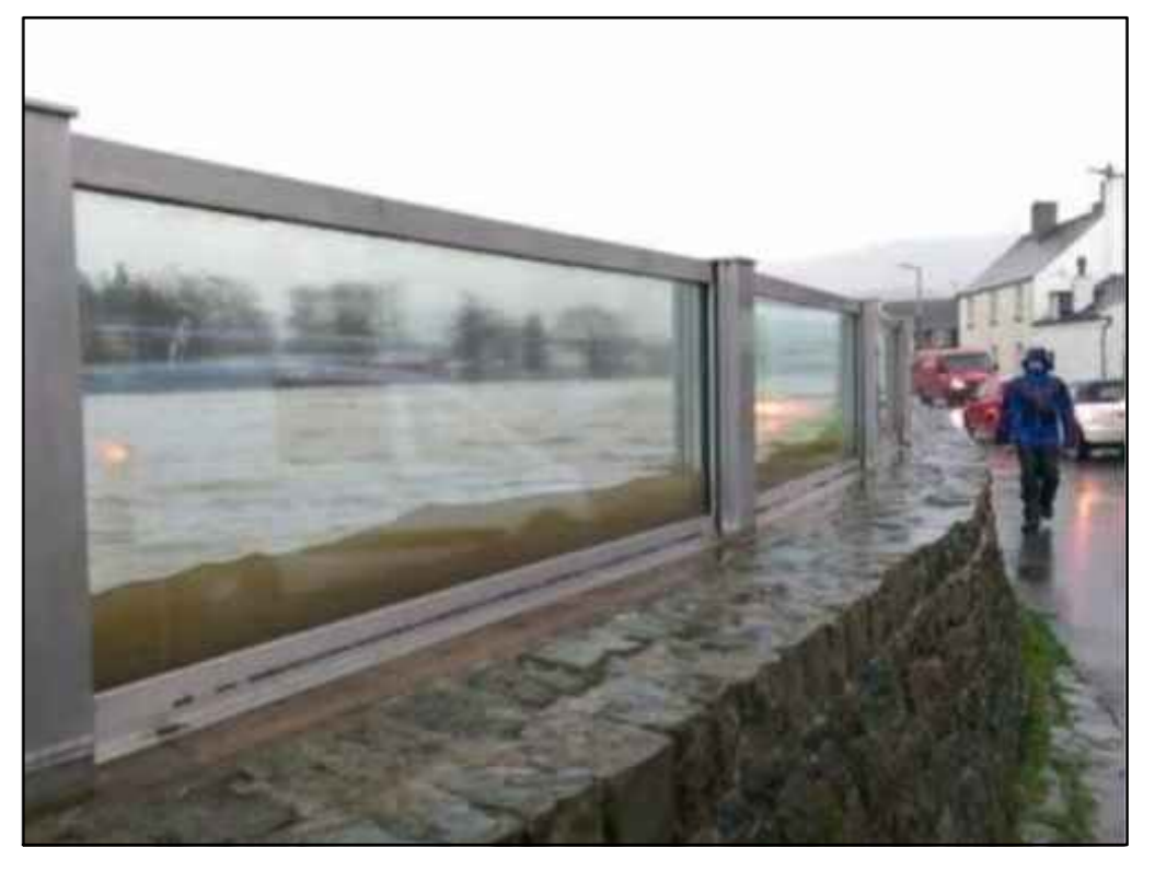
EXAMPLE OF EXISTING STONE WALL WITH TOP MOUNTED GLASS AND STAINLESS STEEL FLOOD PROTECTION (RIVER GRETA, KESWICK)
