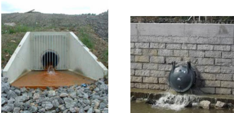
Figure 3.2 Typical storm water headwall in an embankment with a safety grill and a typical storm water discharge pipe in a wall with a flap valve (reference: http://www.cpm-group.com/products/water-management/stormwater-management/stormwater-control/spillway-outfall ; http://www.focalvalves.com/a/product/Flap_Valve/105.html )
