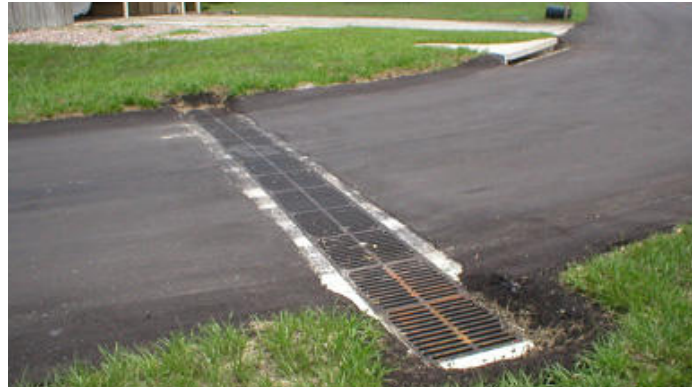
Figure 3.11 Example photograph showing heavy duty large volume drainage channel constructed across a street (reference: http://eric-sons.com/roadway.html )
